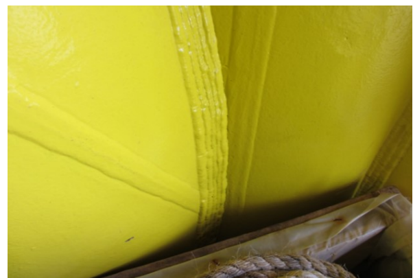
Figure 2: Weld on W and Weld Proximity Identified During Inspection
