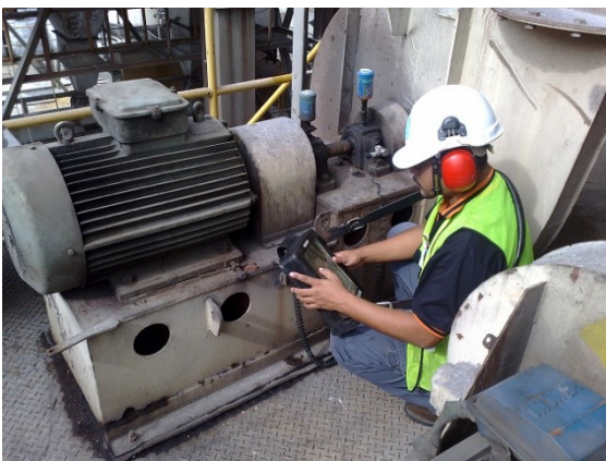
Figure 1: Vibration analysis of motor & fan impeller at Shah Alam, Malaysia
