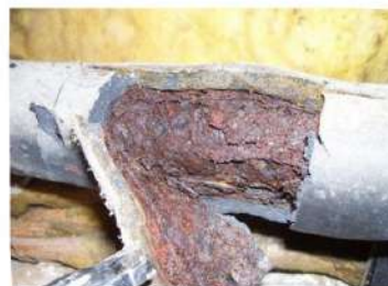
Figure 2: CUI exposed under insulation
