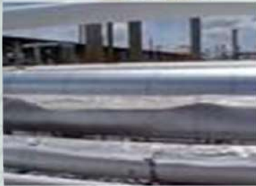
Figure 4: Personnel stepping on and damaging the cladding
