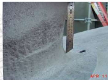
Figure 3: Wall thickness loss due to CUI
